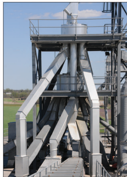
Modified Rapat distributor with enlarged spouting (middle platform) below a second, new Rapat distributor (top platform). Photo by Tucker Scharfenberg.
